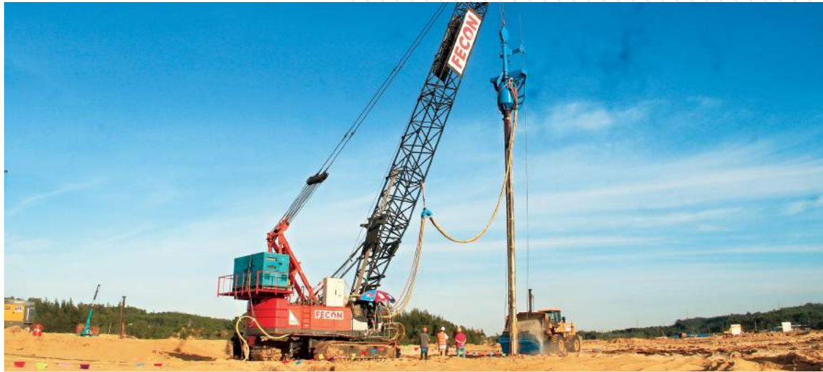
Hoa Phat Dung Quat Steel Factory (Quang Ngai) - Vibro compaction and vibro replacement
