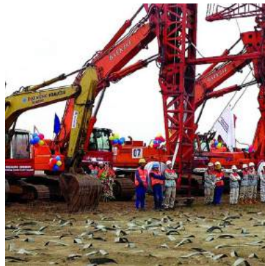
Pic 3 + 4. Thai Binh Thermal Power- Soil improvement work by PVD installation combined with vacuum pre-loading method
