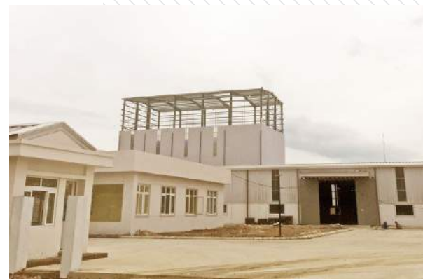
Cristobalite Material Factory (Hue) - General contractor of reinforced concrete structures and steel frames.
