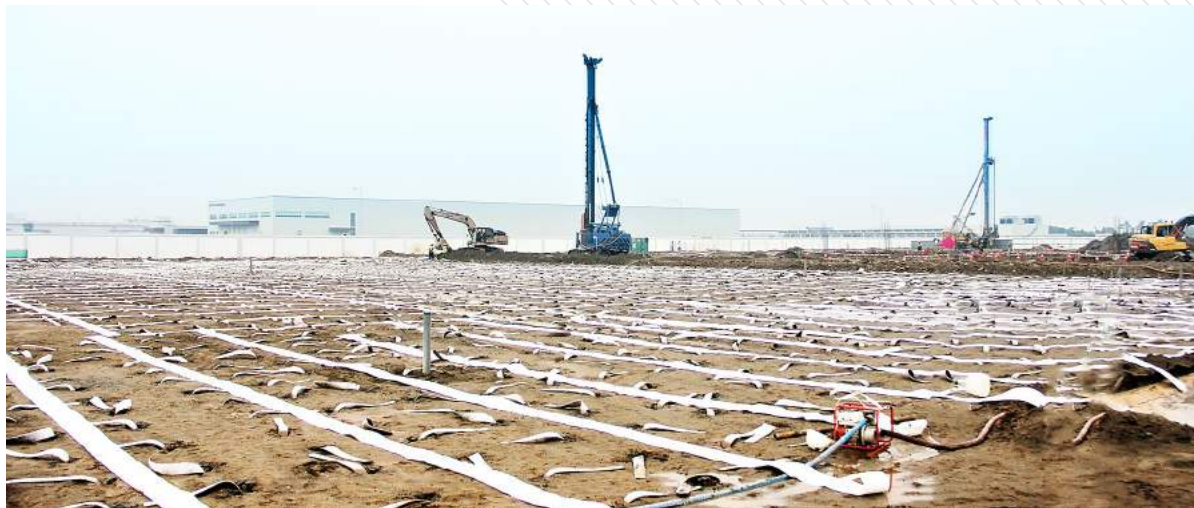
LG Display Hai Phong factory - Soil improvement by PVD Installation & DCM method: 50,234m50.234m
