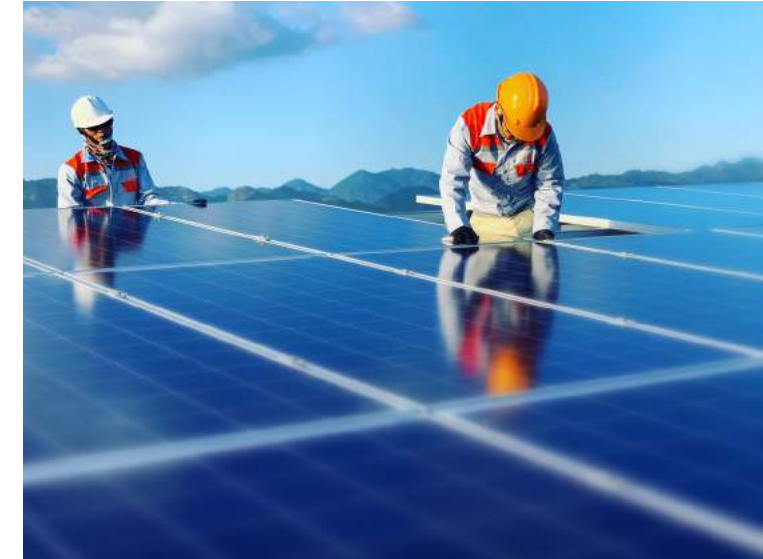
Vinh Hao 6 - Solar Power Plant
