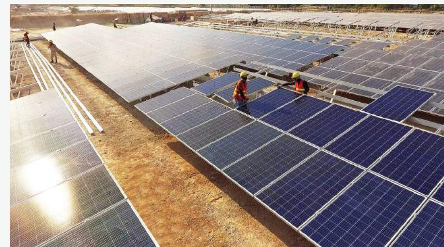
▲ Pic. Vinh Hao 6 Solar Power Plant (50MW)
