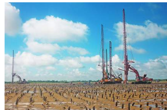
Long Phu 1 Thermal Power Plant
