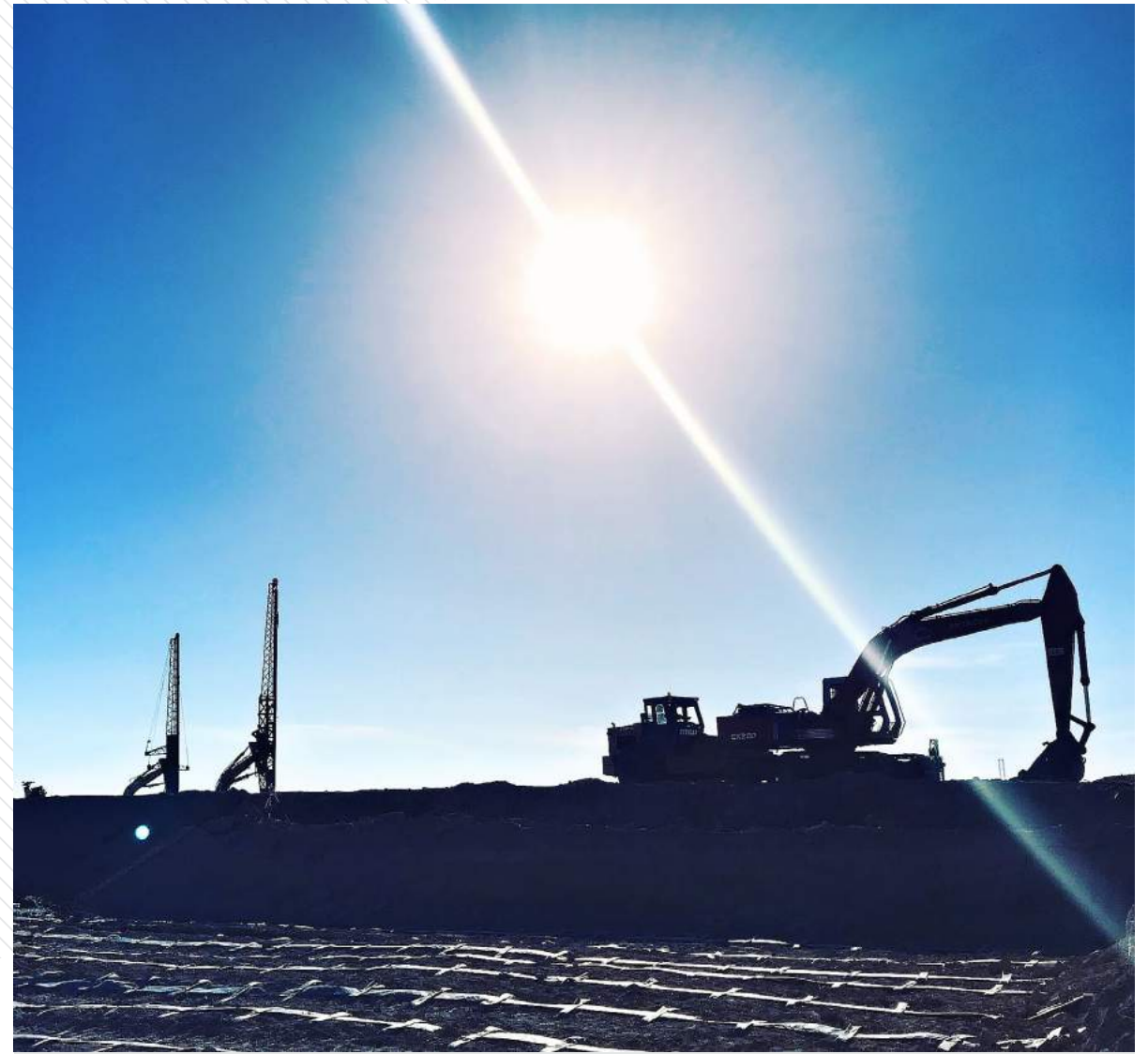
Long Son Oil Refinery Plant (Ba Ria, Vung Tau) - Soil improvement by PVD installation and Vacuum pre-loading method, Dynamic Compaction
